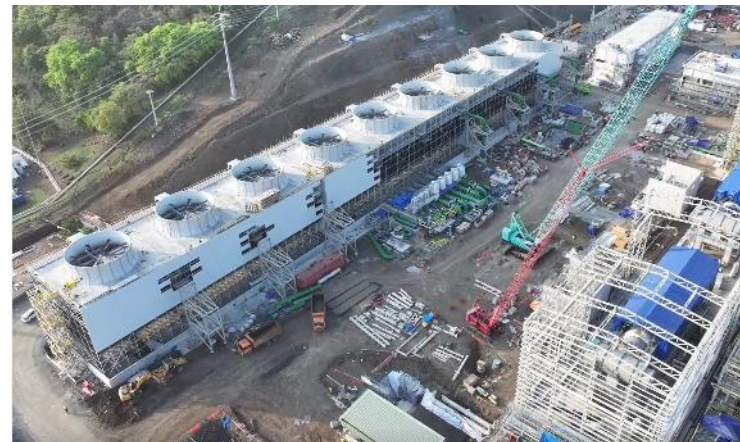
Steam Turbines and Cooling Towers
