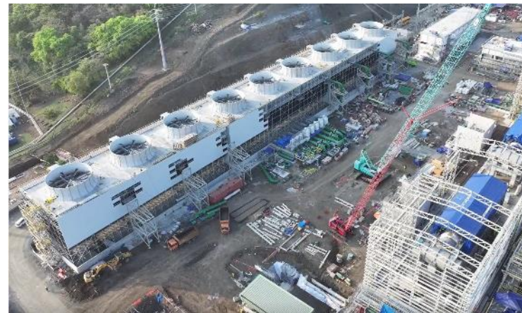
Steam Turbines and Cooling Towers
