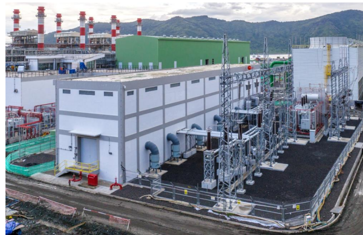
GIS and Switchyard
