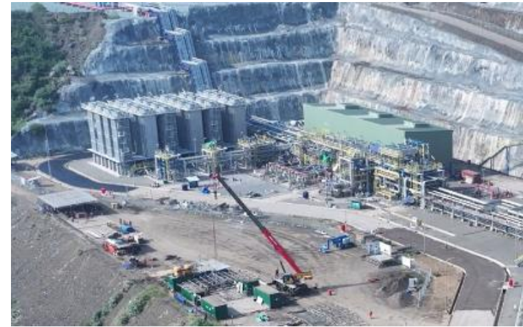
Ambient Air Vaporizers (AAV) area
