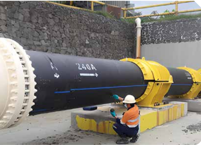
Monitoring of Deep Sea Tailings pipeline thickness
