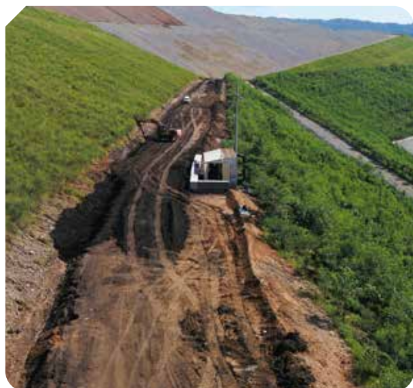
^ The process of FABA utilisation as a road base include (1) mixing FABA and soil (2) application of the mixture onto the road and (3) compaction of the mixture.
