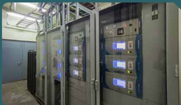
^ CEMS Analyser rooms at AMMAN's power plant.
