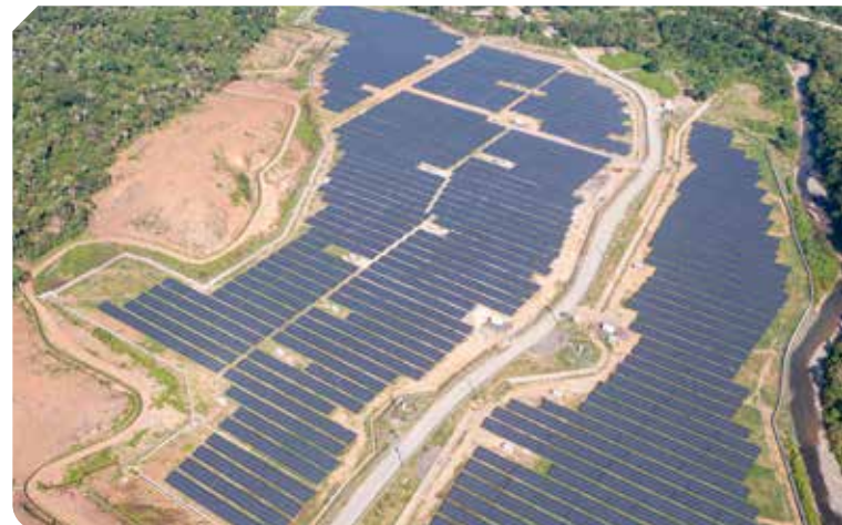
▲ The Sumbawa Solar PV Power Plant will supplement electricity supply to our processing plants and substations, paving the way for a cleaner and greener future.
