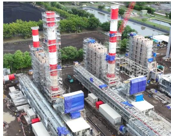
Two Gas Turbines
