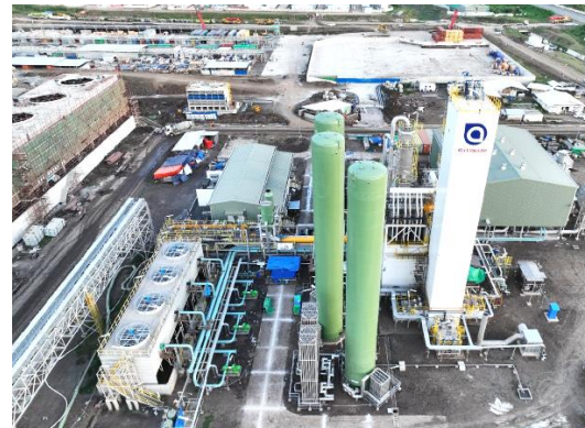
Air Separation Unit
